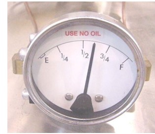
Differential Pressure Gauge (1)
